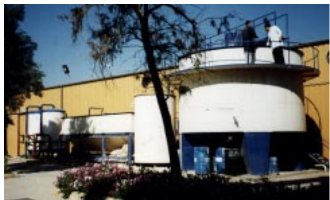
Industrial effluent (waste) water treatment from dye house plant
