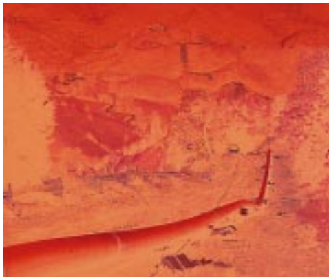
Construction of the TransGas de Occidente pipeline in Colombia. We have a 34% interest in and operate this natural gas pipeline – a 344 km pipeline with 400 km of laterals. The line crosses some of the most difficult mountain terrain in Colombia.
